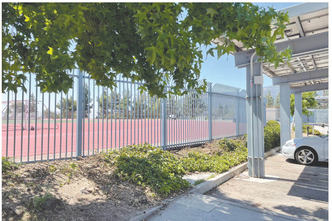
Construction has already started at CV High School with the installation of new fencing. Photo by Mary O'KEEFE
